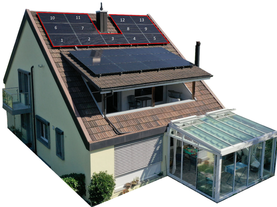
Figure 4. Single-family home with residential PV system (modules with 3 bypass diodes) and shading objects of type chimney and ventilation pipe. The 13 kWp PV plant was implemented by PV installer in Switzerland. Reproduced with permission. [30] Copyright 2022, Alsona AG.
