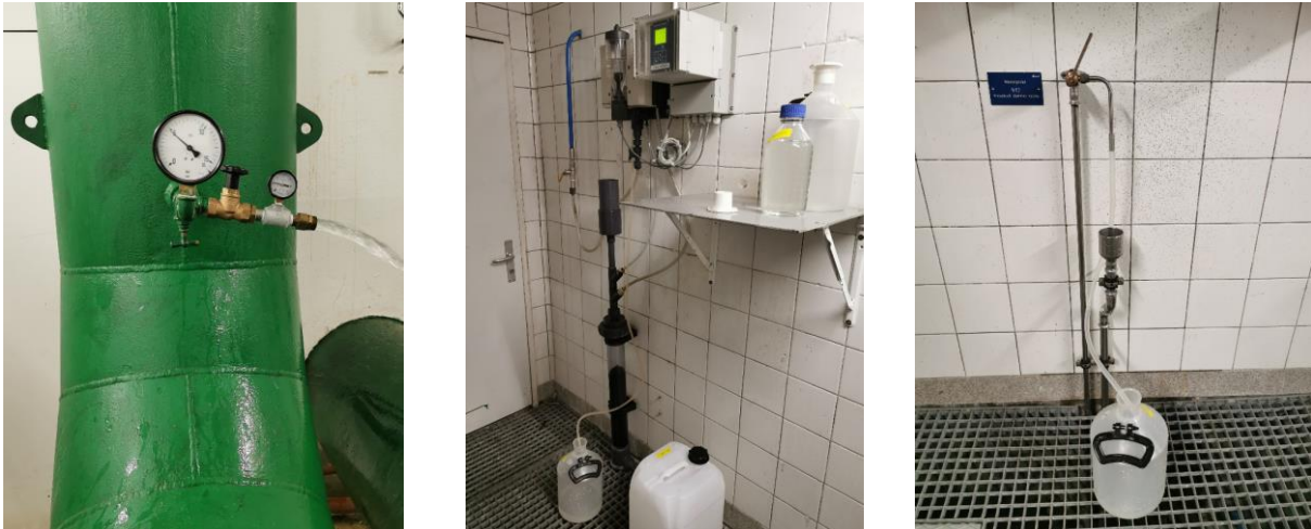
Figure 6: From left to right; Raw water from lake Vierwaldstättersee; Sampling for water after ozonation; Final treated water before distribution. (Source: Erb Severin)
