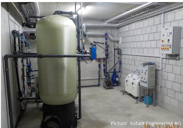
Figure 8 Plant room with two PSF, AOP and all electrical equipment Source: Autark Engineering AG
