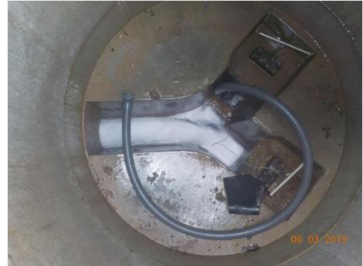
Figure 13 High flow of laundry wastewater from pumping pit Source: Autark Engineering AG
