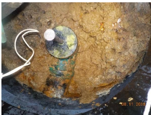
Figure 15 Septic tank inlet filled with scum
