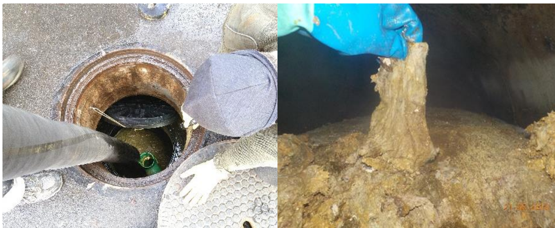
Figure 21 Pumping out of first chamber of septic tank (left), wet wipes clumped with scum (right) Source: Pravin G.Moorthy
