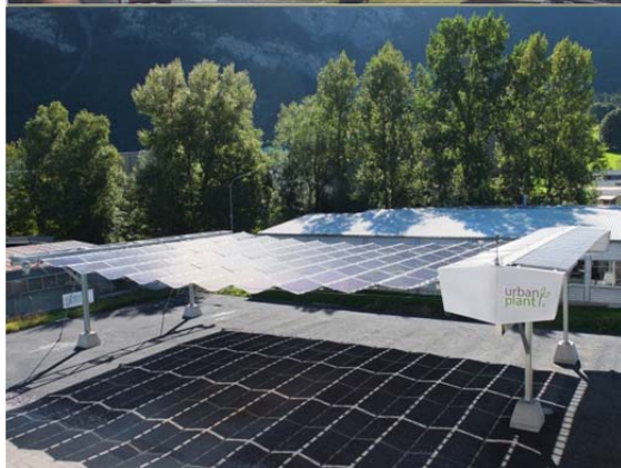
Figure 7: Urban Plant UP50 Prototype operating since June 2013 (16m x 25m and 54kWp).
